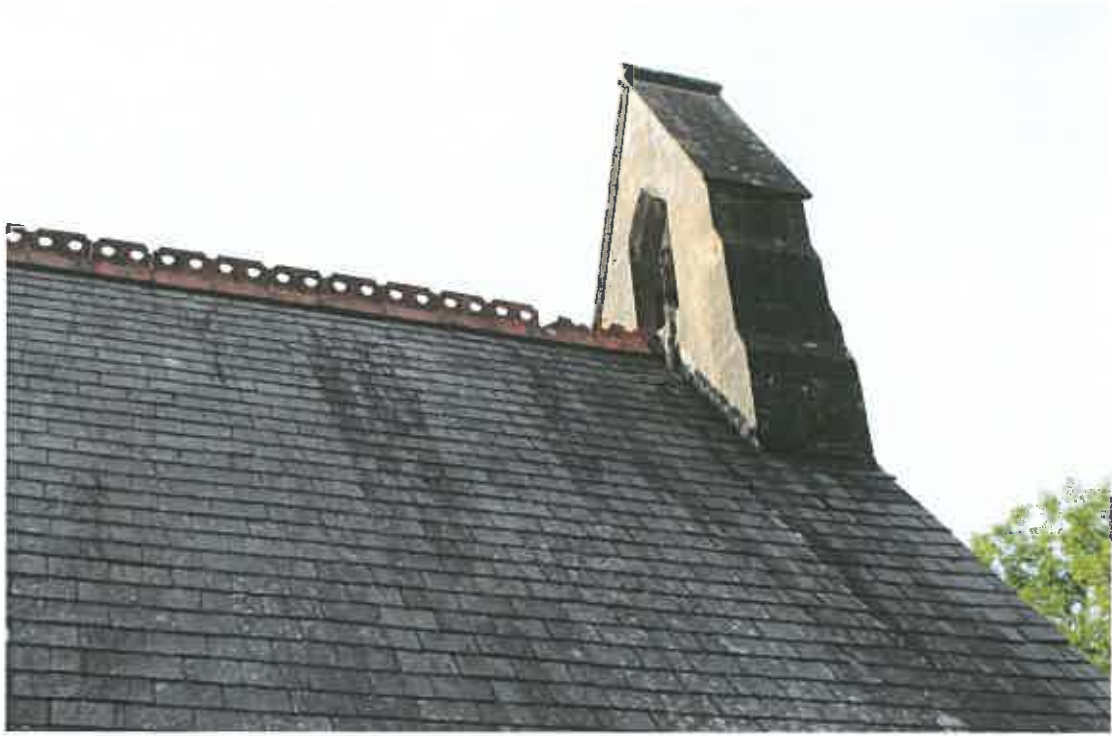
Broken ridge tiles beside the bellcote.
