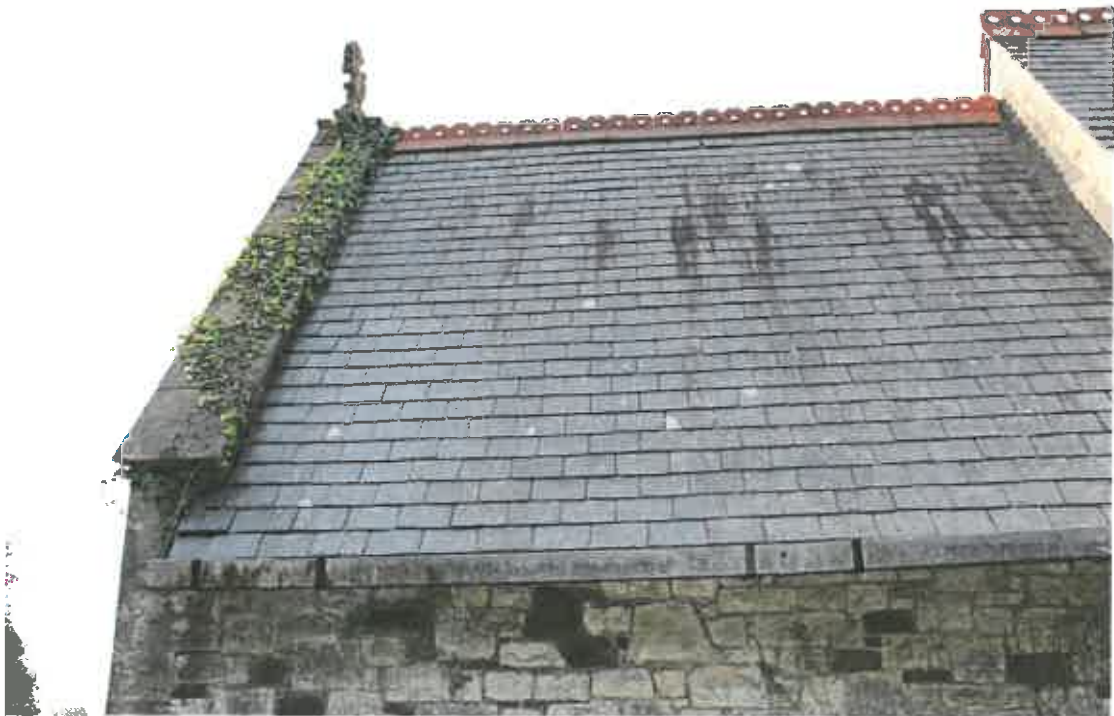
Plant growth on the North slope of the East gable. Rainwater gutter rusting and in need of painting.
