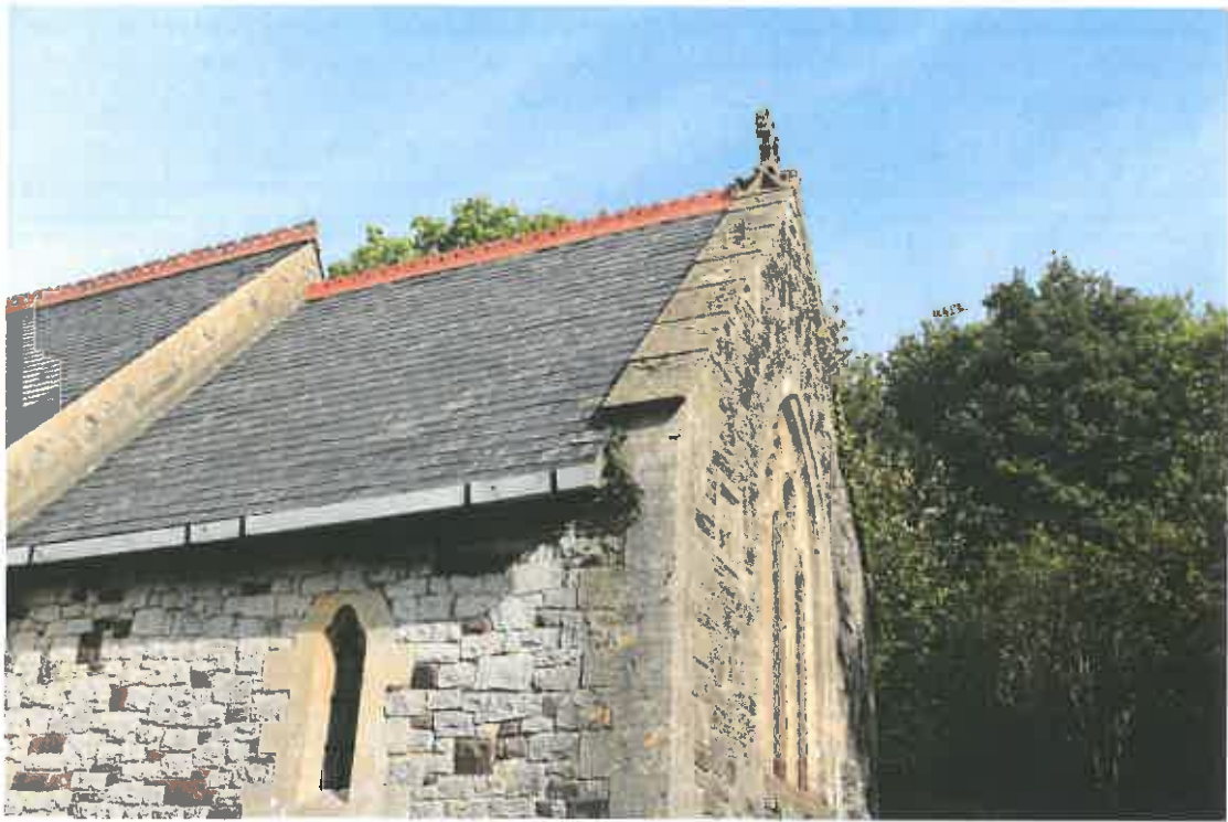
Plant growth at the South East corner and repointing needed under the ridge tiles.
